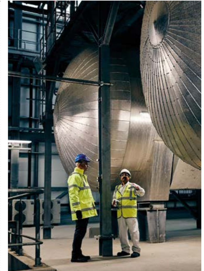
The two feed water tanks at Riverside have a capacity of 150m 3 each and an operating level of 80m 3 .
