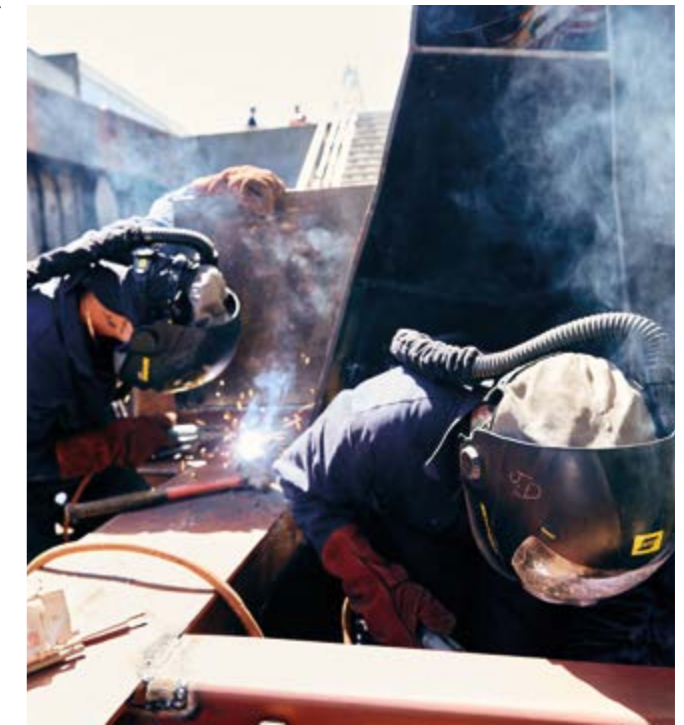
Welders at our Charlton Barge Yard oversee the maintenance of our vessels.
