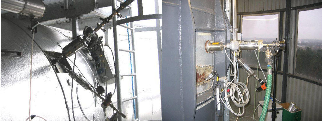
Figure 10. Fine particle measurement from duct between filter and stack at Kauttua (on left) and from the stack at Norrköping (on right).
